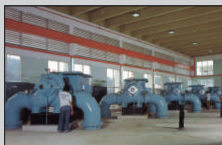
Splitcase pumps at Sungai Langat, Malaysia
