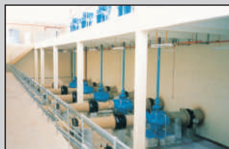
Pelubang Water supply project ALOR Setar Kedah, Malaysia
