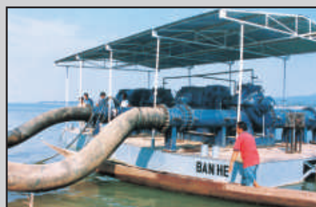
Pontoon mounted splitcase pumps at Banhe, Lao PDR
