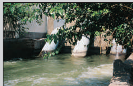
Tahdy 'C' canal water pumping station, Egypt
