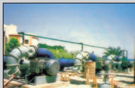
Mixed Flow pumps for sewage application at Faiyad, Egypt
